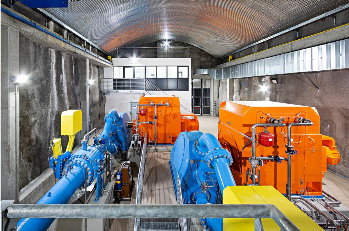
Power plant "Maisonettes", Valle d'Aosta, Italy, Year 2020
